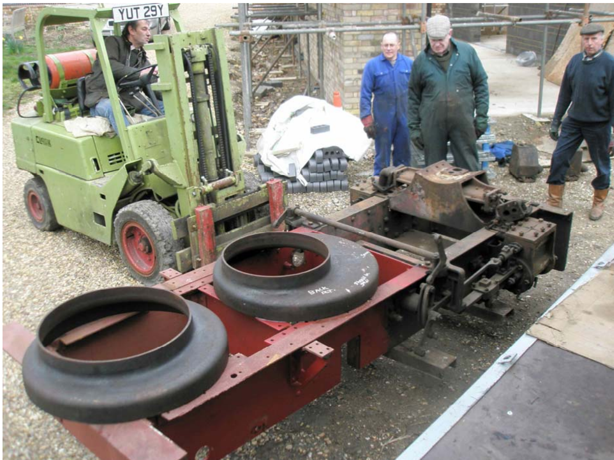
Loading the complete frames into the ERF, the new backhead and throat plate are on top. Note the complex smokebox saddle casting; this will likely have to be made new in order to convert to 2ft gauge! Steve Bell
